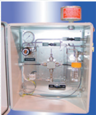
Extractive flow cell with heated SHS, pressure regulation, and calibration
